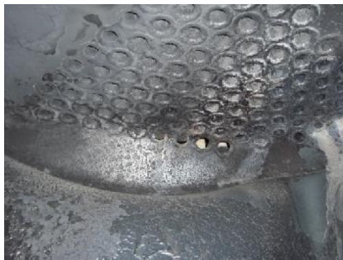
View from Burner Opening
