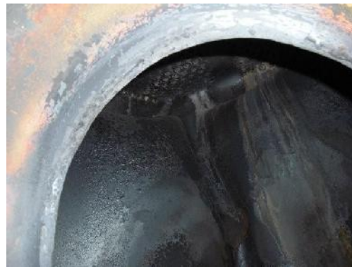
View of Deformed Top TubePlate
