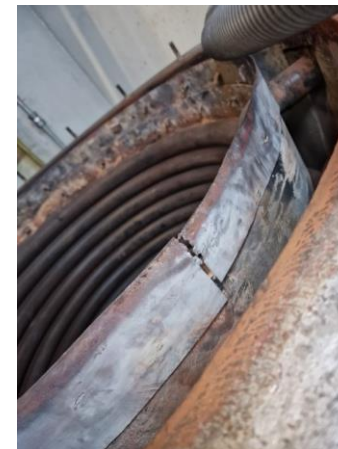
2. Steel parts to be repaired by welding
