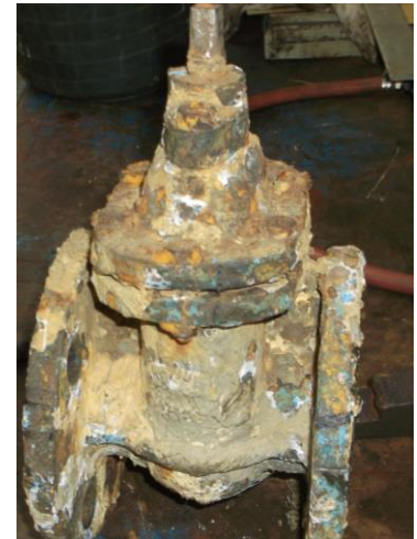
Engine room valves status
