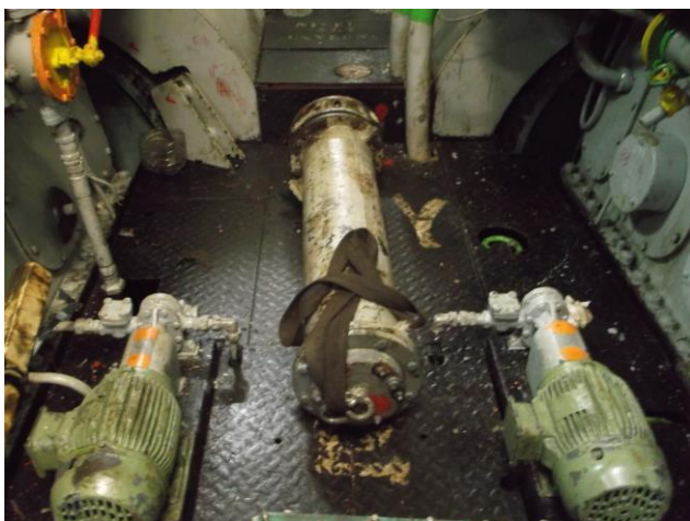
Coolers and pumps in ER
